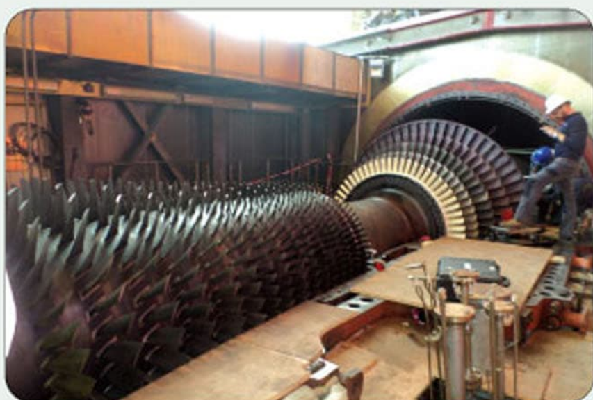
C1 Inspection of Khulna 150 MW PPP : View of Compressor & Turbine
