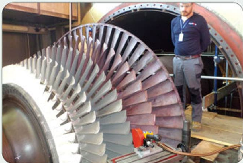
C1 Inspection of Khulna 150 MW PPP : View of Gas Turbine
