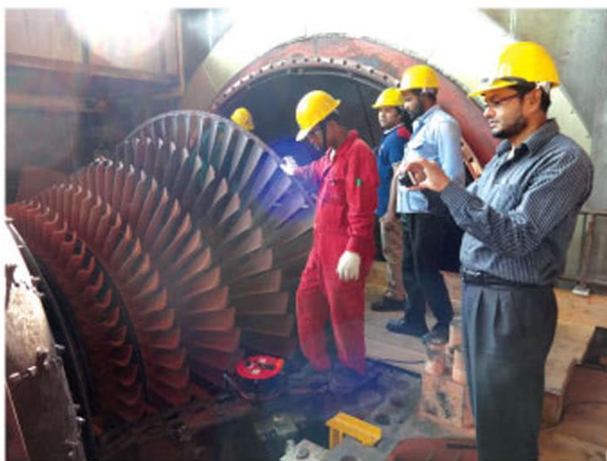
C1 Inspection of Khulna 150 MW PPP : View of Gas Turbine
