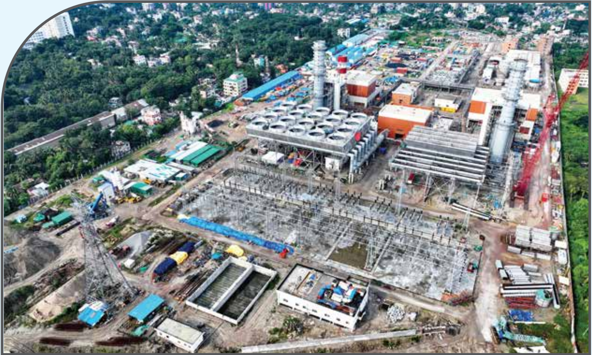
Rupsha 800 MW Combined Cycle Power Plant Project
