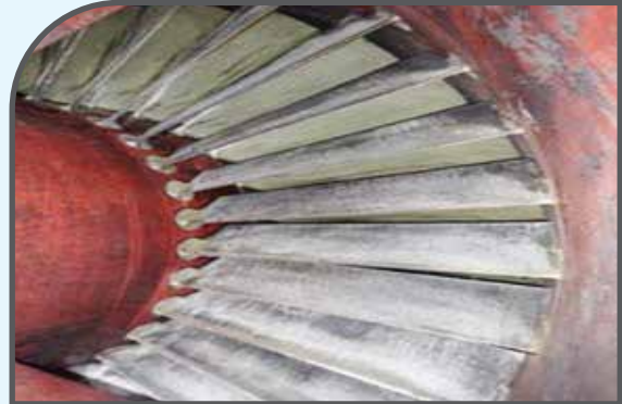
Borescopic Inspection of Gas Turbine of Sirajganj 225 MW CCPP Unit-1 (7 Jul 2023 to 12 Jul 2023)
