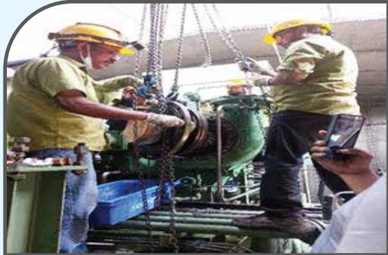
Major Overhaul of Gas Booster Compressor (GBC)- 1& 2 of Sirajganj 225 MW CCPP Unit-1 (13 Mar 2023 to 21 Mar 2023)
